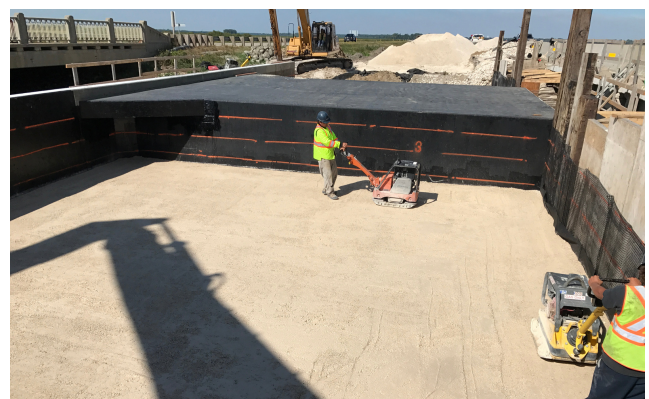
Lower-layer lift of granular over the Pyramid Grid™ being compacted. The orange lines represent the layers/thickness of granular to be placed over the grid.
