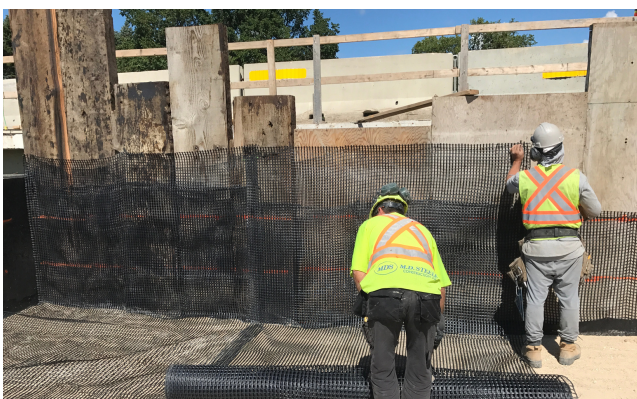
Deployment of the Pyramid Grid™ with the importance of extending the grid in each layer as an overlap.
