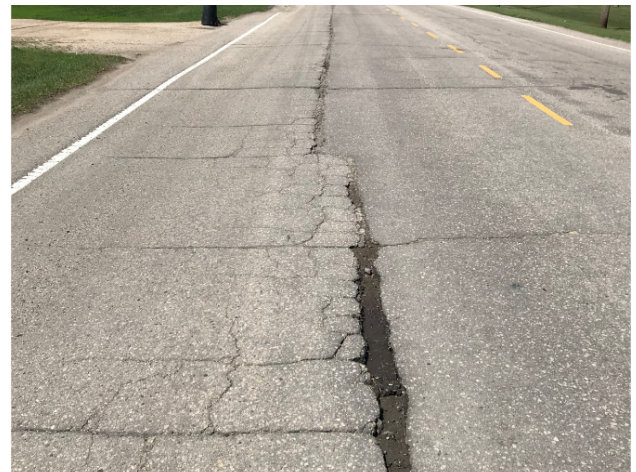
Before construction showing significant fatigue in road.
