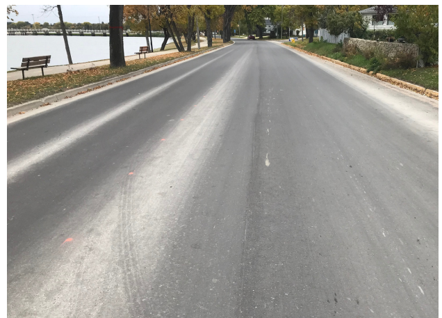
Construction with Spartan Road Grid™ 10 - 1 year after with no signs of cracking or fatigue.
