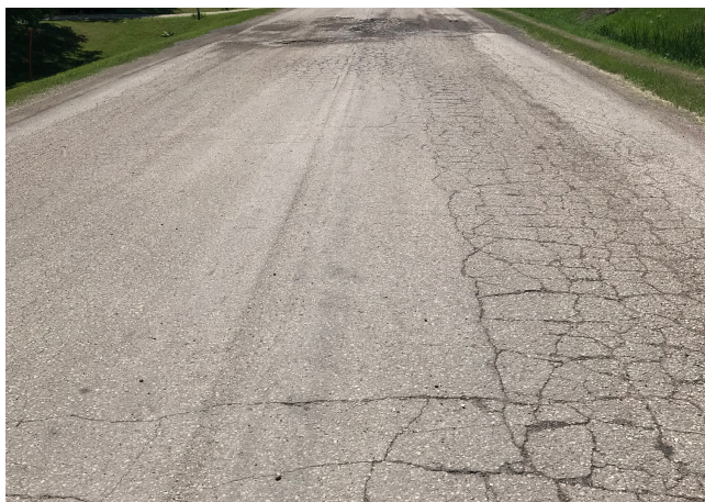
Before construction showing significant fatigue in road.
