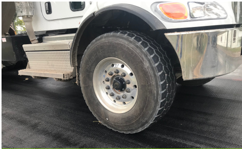
Heavy equipment tire on top of grid with no sticking or lifting of material.
